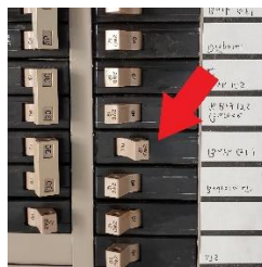
The breaker is off.
