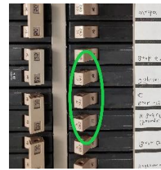
These breakers are on.
