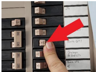
A tripped breaker will be between off and on.
